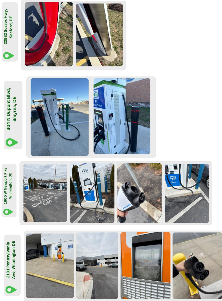
Figure 3. 7. Photos of Public EV Charging Station Conditions
